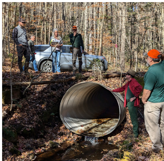
A perched and undersized culvert in the Moose River Plains is evaluated by DEC and Trout Unlimited partners for rightsizing.
